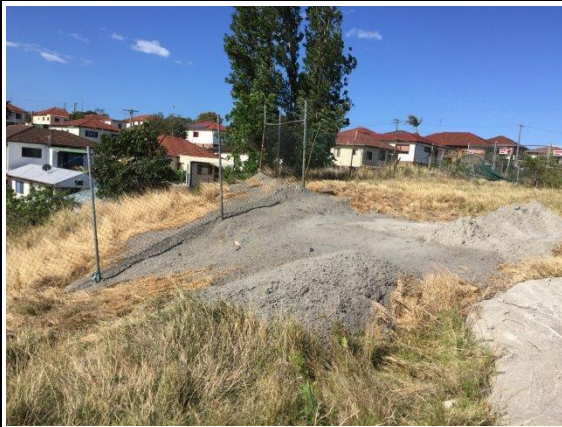
Photo 7. Initial Site Assessment - 31 st October 2017 - Area of Concrete Pad and internal fence covered with wet sand
