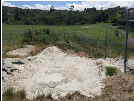
Photo 17. Installation of permanent Temperature Probe - (300mm depth) - 28 th November 2017 - internal northern fence line
