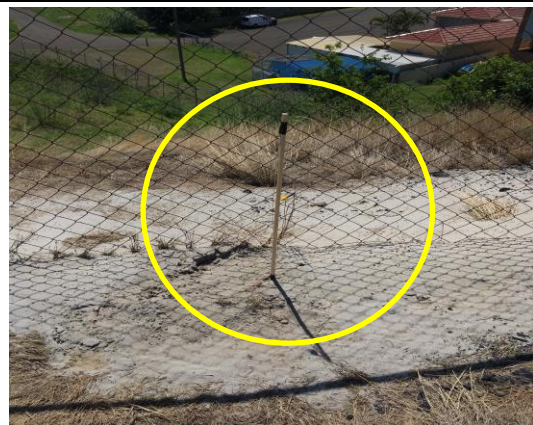
Photo 16. Installation of permanent Temperature Probe - (300mm depth) - 28 th November 2017 - internal northern fence line
