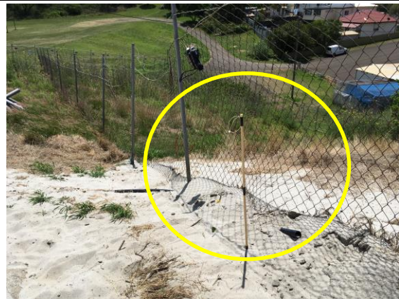
Photo 18. Installation of permanent Temperature Probe - (300mm depth) - 12 th December 2017 - internal northern fence line
