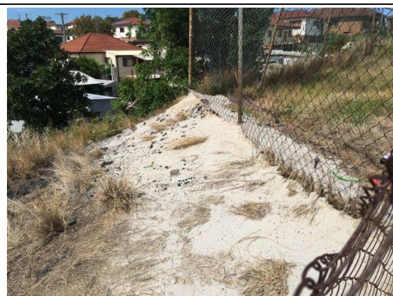
Photo 14. Hand-held Temperature Probe - Surface (150mm depth) - 24 th November 2017 - internal northern fence line
