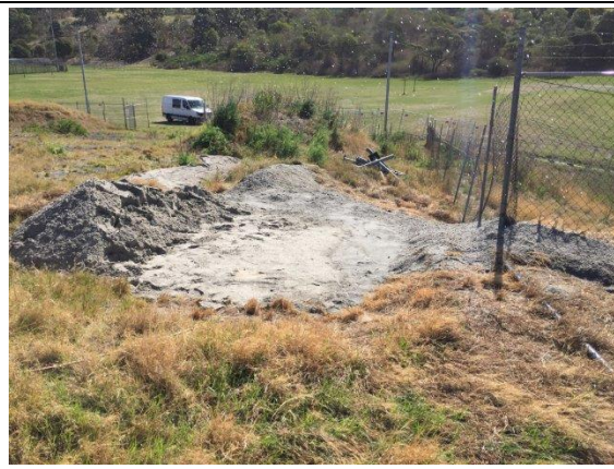
Photo 6. Initial Site Assessment - 31 st October 2017 - Area of Concrete Pad and internal fence covered with wet sand
