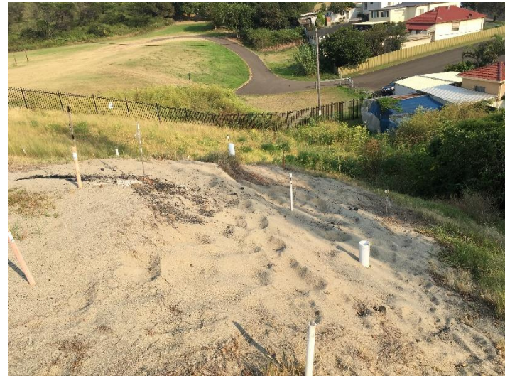
Picture 2 – Slope within north-western hotspot area
