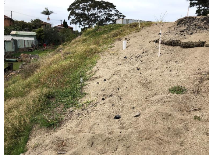
Picture 2 – Slope within north-western hotspot area
