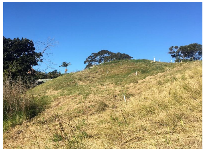
Picture 4 – Slope within north-western hotspot area
