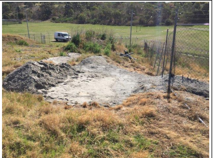
Photo 4. Initial Site Assessment - 31 st October 2017 - Area of Concrete Pad covered with wet sand
