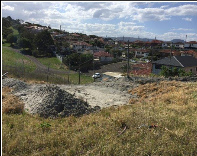
Photo 3. Initial Site Assessment - 31 st October 2017 - Area of Concrete Pad covered with wet sand
